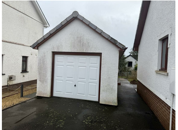
Detached garage with front up and over door and rear courtesy door.
